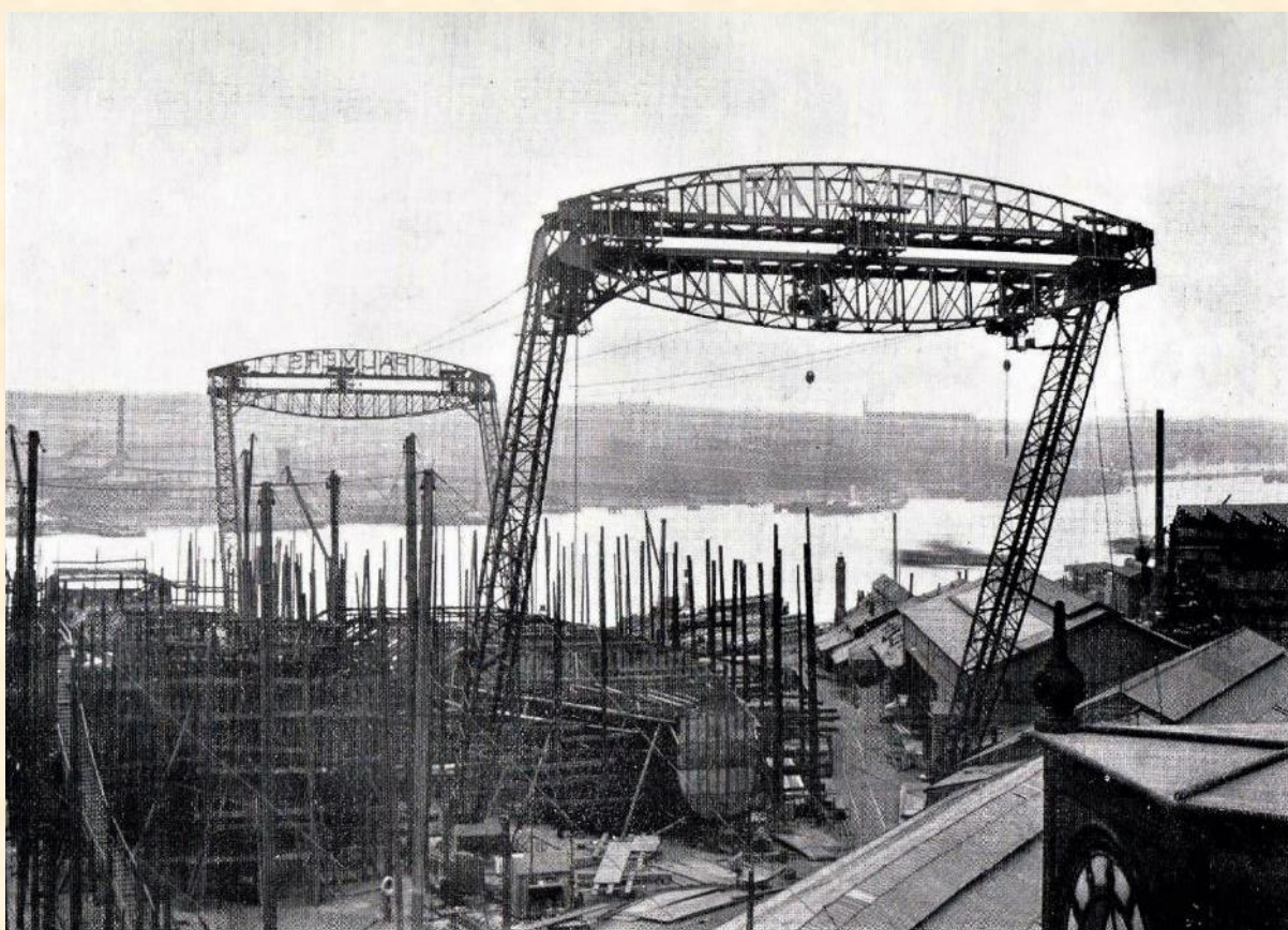
Electric overhead trolley cranes with elliptical gantries, standing 135 ft (41 m) on 'sheerlegs' above the berths at Palmers shipyard in Jarrow. These were installed in 1906 to speed up production. (From Some Account of the Works of Palmers Shipbuilding & Iron Co Ltd by Malcolm Dillon, Co Secretary; fourth edition, 1909; with thanks to John Bage)
